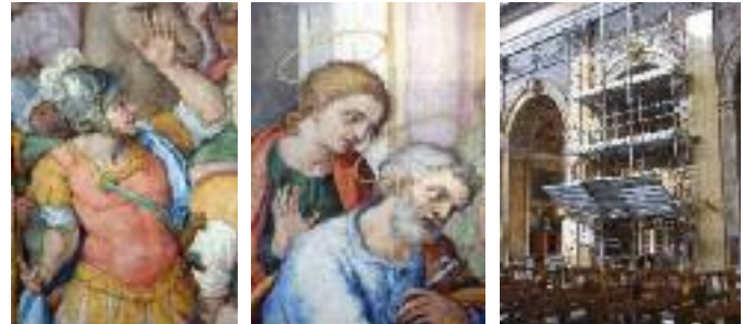
Restoration interventions by our students at the Church of Santa Maria in Traspontina in Rome
